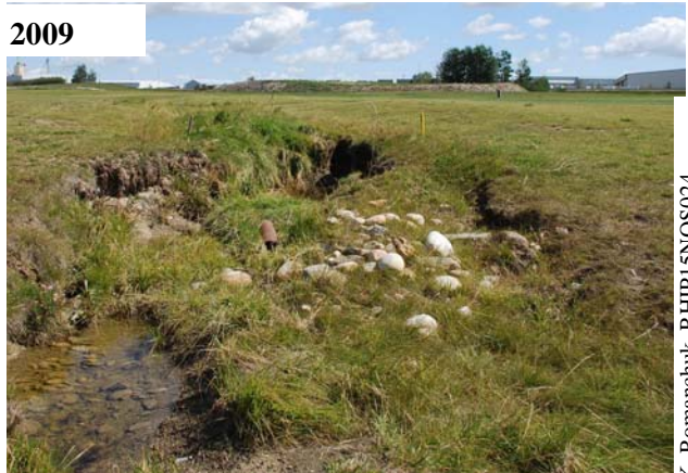
NOS15D Erosion along a small tributary that flows into Nose Creek near the upstream end on the east side of the creek. Lack of a riparian buffer is contributing to erosion.
