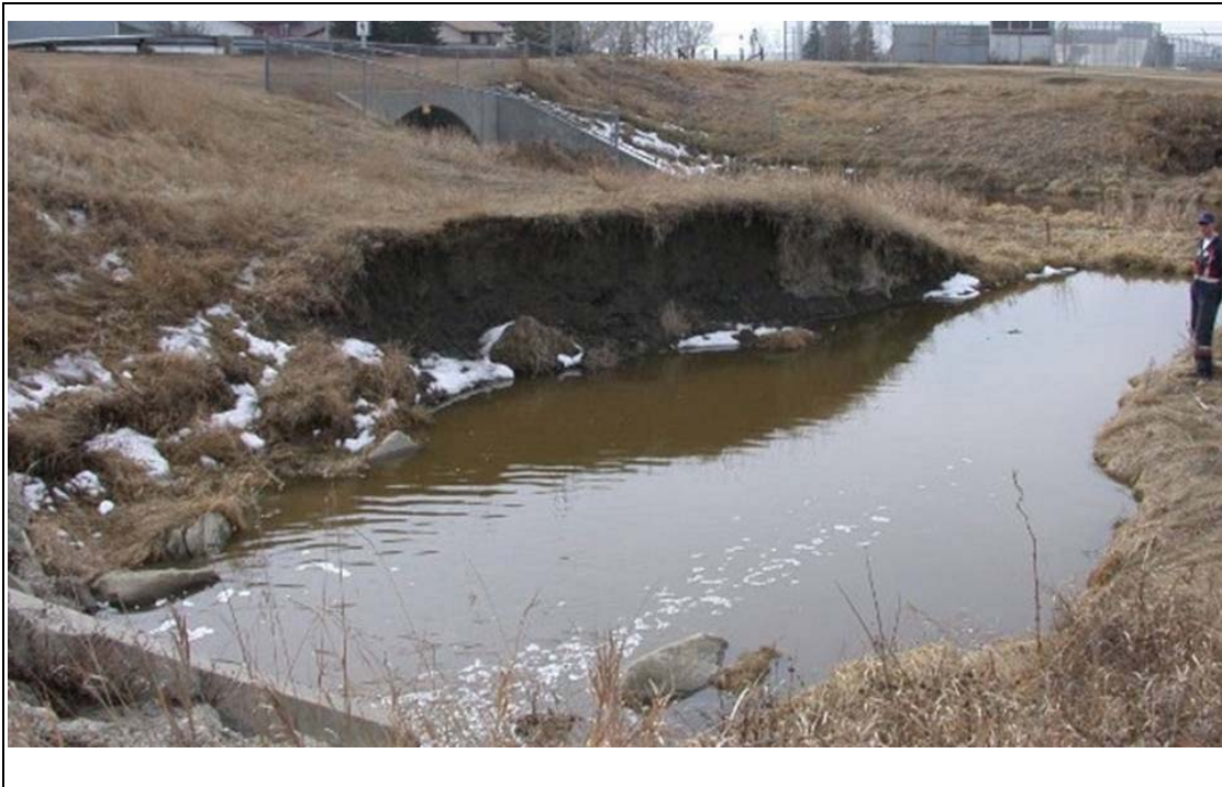
Photo w: Pre-restoration photograph (2006), showing eroded bank downstream of a stormwater outfall at the downstream end of the Nose Creek Park riparian inventory site.
