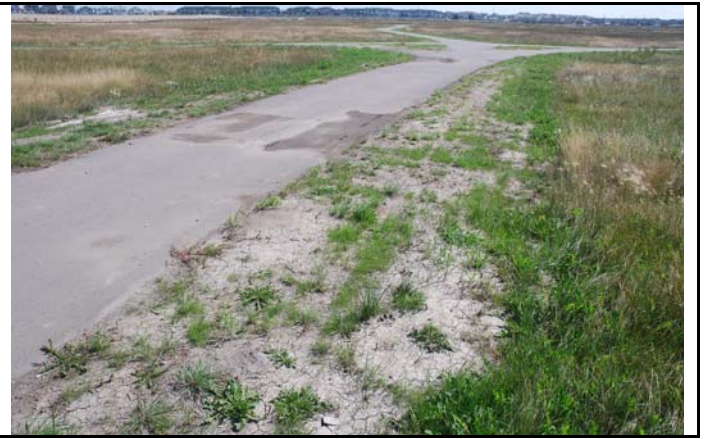
Photo h: Bare ground adjacent to recently constructed paved trails in the Williamstown Reserve has been seeded with a native seed mix, but it also has good potential for natural recovery. (Photographer: K. Hull, Catalogue Number: RHIP22NOS012).
