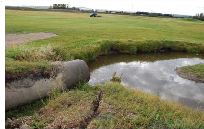
Photo i: Bare ground has resulted from erosion of this culvert crossing in the golf course site. Soil compaction and landscaping due to fairway developments have caused streambank and floodplain alterations. (Photographer: K. Romanchuk, Catalogue Number: RHIP15NOS023).
