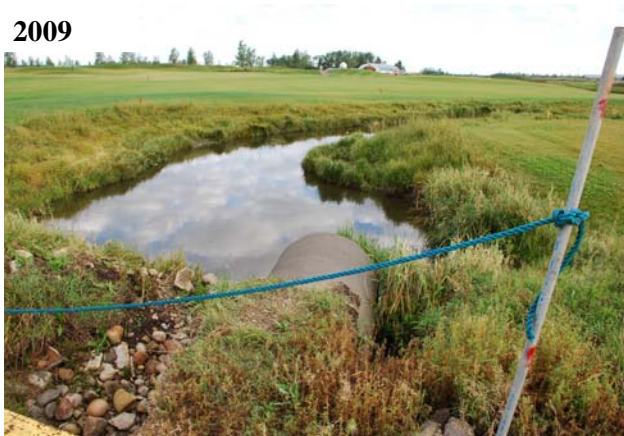
NOS15A Culvert crossings constrict water flows creating ice jams, erosion and bank slumping. This increases sediment inputs into the stream, decreasing water quality.
