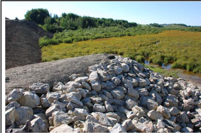
Photo s: New road construction along the south end of the Rocky View Environmental Reserve. Rip-rap has been installed at the culvert. Roads and culverts have potential to alter natural subsurface and surface hydrology. Long-term monitoring is suggested to examine these effects. (Photographer: K. Hull, Catalogue Number: RHIP07WNO013).
