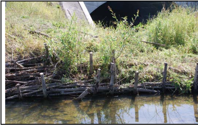
Photo g: Live willow cuttings and wattle fences were installed along this eroded bank in 2006 as part of a soil bioengineering workshop. This portion of bank is located adjacent to a stormwater outfall at the downstream end of Nose Creek Park in Airdrie. (Photographer: K. Hull, Catalogue Number: RHIP04NOS020).
